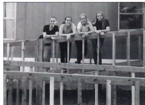
Nucla High School students worked in collaboration with Len Spina, the school and Tri-County Health Network to compete construction of a wheelchair ramp for one local citizen. (Courtesy image)
